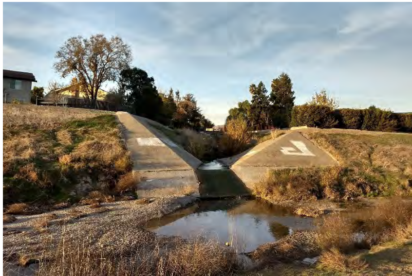
View of side channel, which would need a bridge to continue trail
