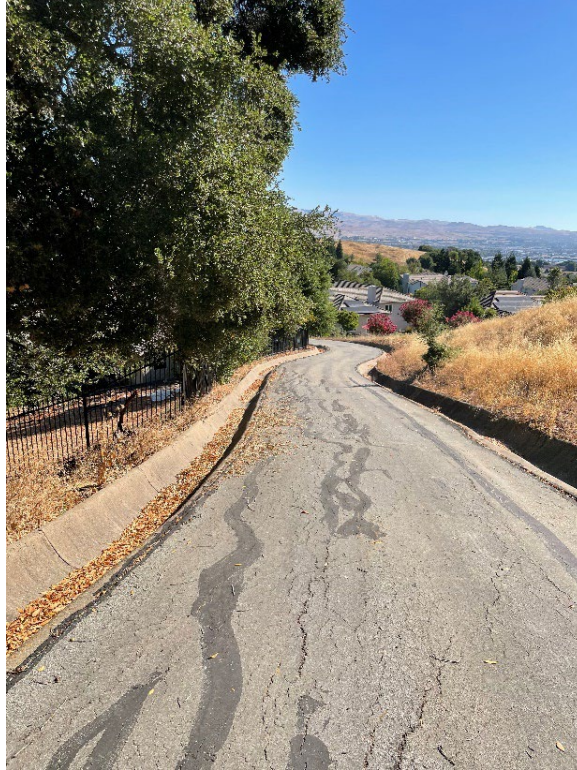
ID LC-22: Cracking and distress on access road.
