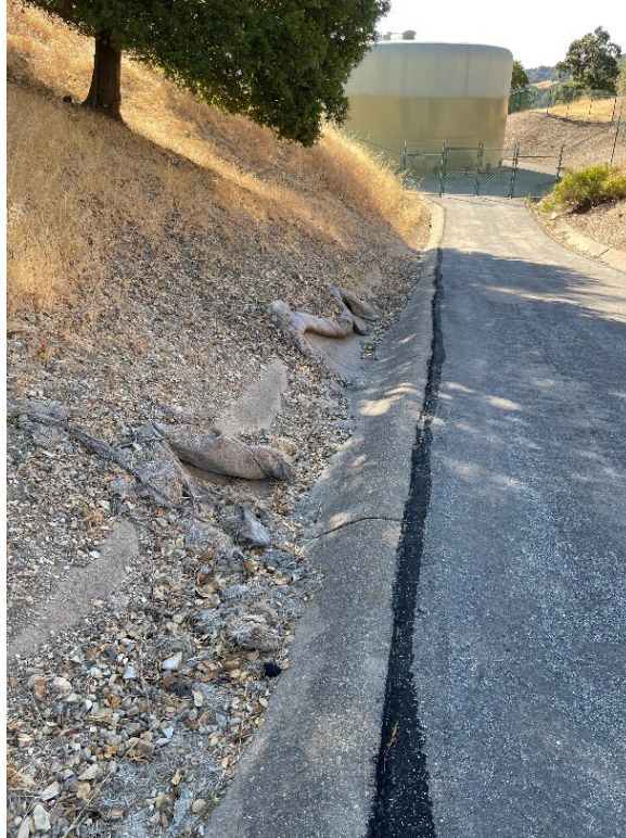
ID LC-39: Straw wattle damaged.
