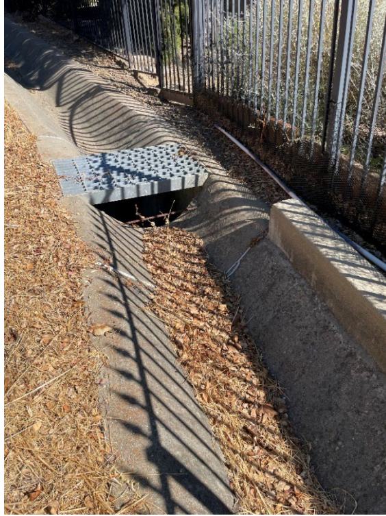
ID OTF-6: Degraded wattle along drainage ditch. Debris in V-ditch
