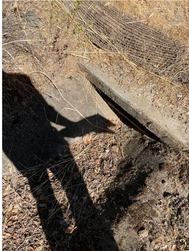
ID OTF-4: Current sandbags runoff directly from private access road above FI#2. Steep Hill
