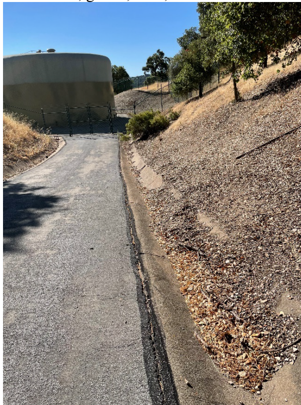
ID LC 40: Debris, gravel, soils, leaves in Concrete V-Ditch
