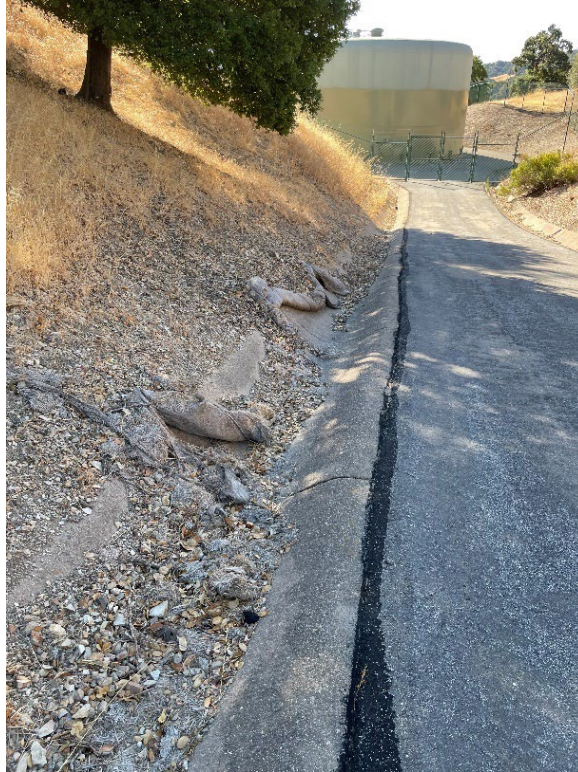
ID LC-39: Straw wattle damaged.
