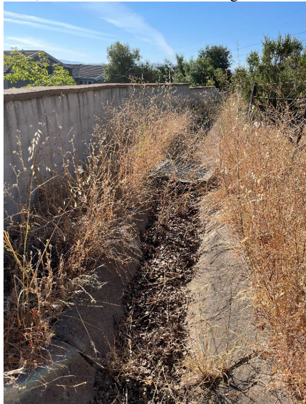
ID LR-18: Debris, weeds, leaves accumulated in drainage ditch. For majority of V-ditch
