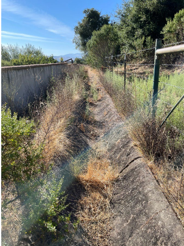
ID LR-17: Overgrown vegetation along drainage ditch.
